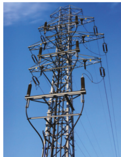
FIGURE 4.1.2 This power transmission tower relies on the strength of iron in steel for its structural integrity. The electricity cables are made from aluminium, utilising its ductility and electrical conductivity.
