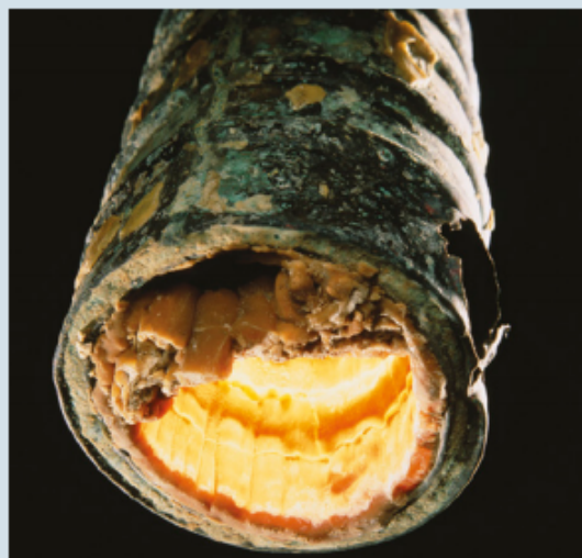
FIGURE 16.1.6 Accumulation of limescale in pipes is a result of precipitation of CaCO 3 .
