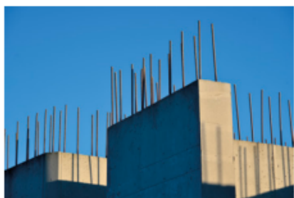
FIGURE 1.1.5 The steel rebar can be seen here embedded in the concrete structure.
